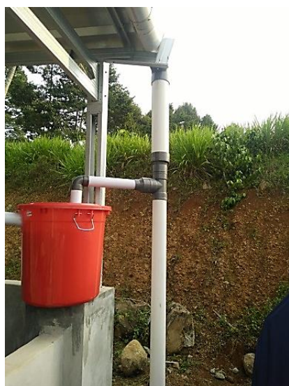
Figure 2. Centrifugal System Installed in Rainwater Harvesting
